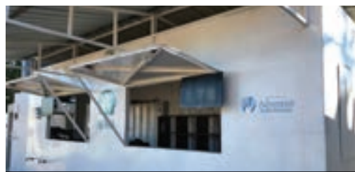
In a GCHM and ADRA partnership, two water kiosks and wells powered by solar energy were installed as pilot projects in Mozambique.—ADRA INTERNATIONAL
